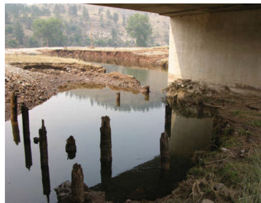
In 2007, flash flooding near Hermosa, South Dakota, caused scouring of bridge abutments at Battle Creek.
