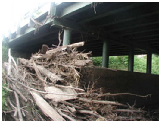
Debris accumulation at a bridge pier diverts flow, enhances contraction, and causes turbulence that contributes to scour of channels and abutments.
